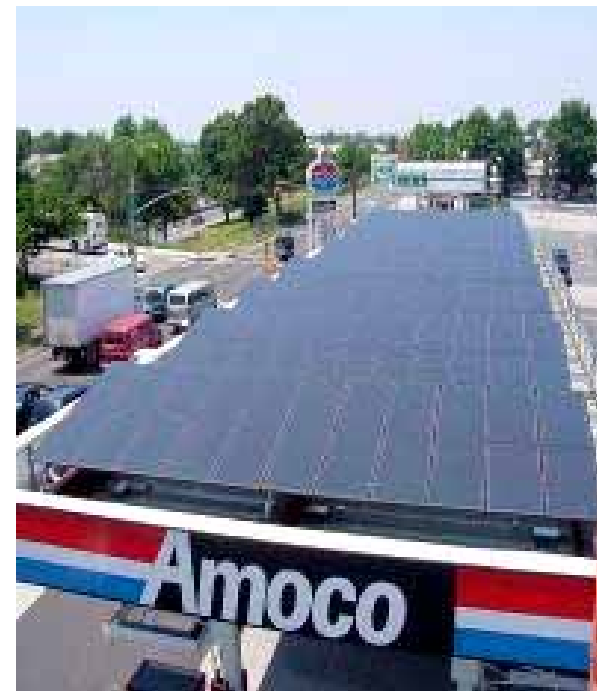
Rack-Mounted Commercial System
