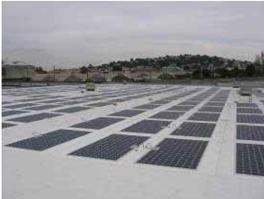
Commercial Membrane System
