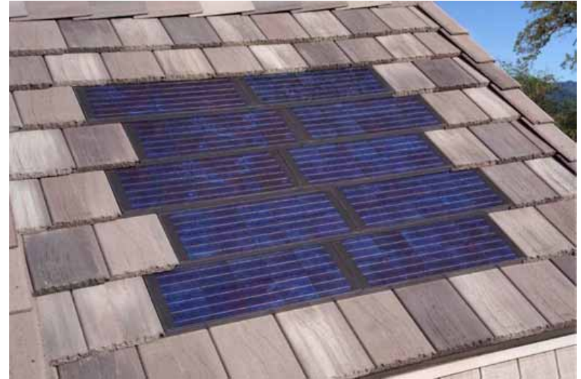
Building Integrated Photovoltaic
