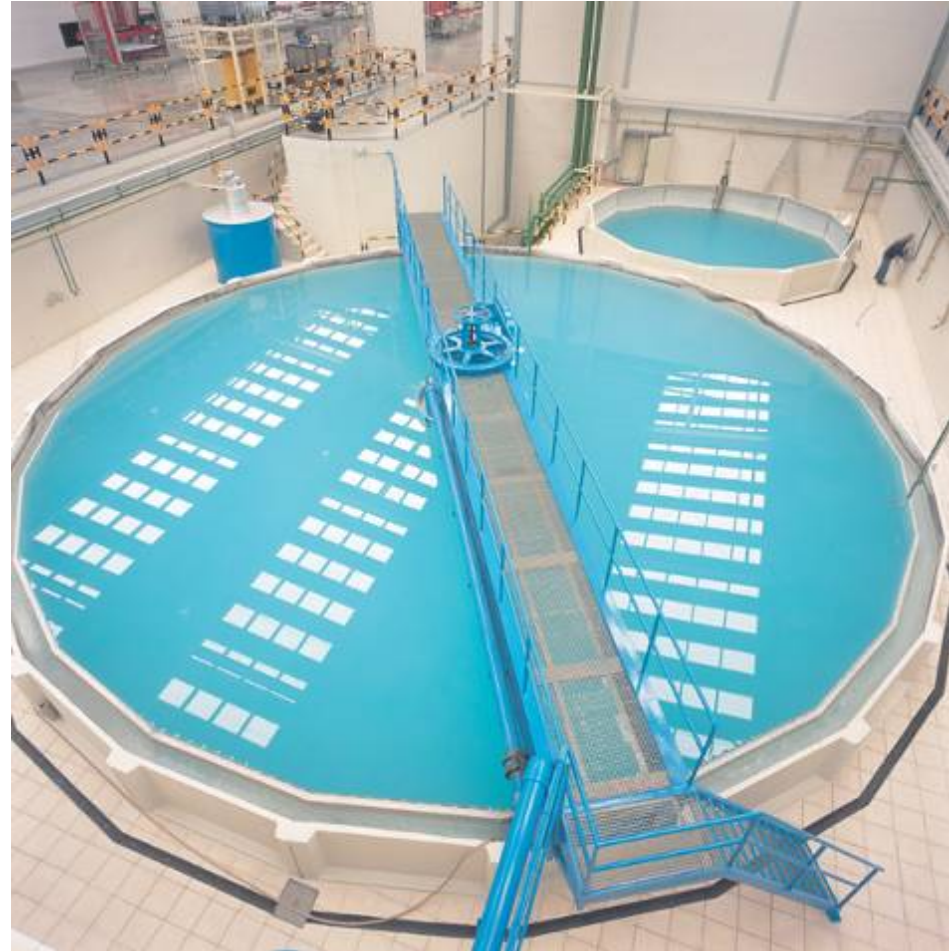
Settlement tanks extract clay particulates and clarify water for reuse
