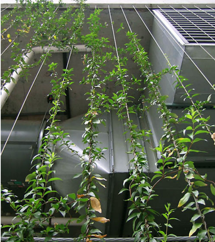
Two-dimensional stainless steel cable system with long vertical spans, Dallas, TX.
