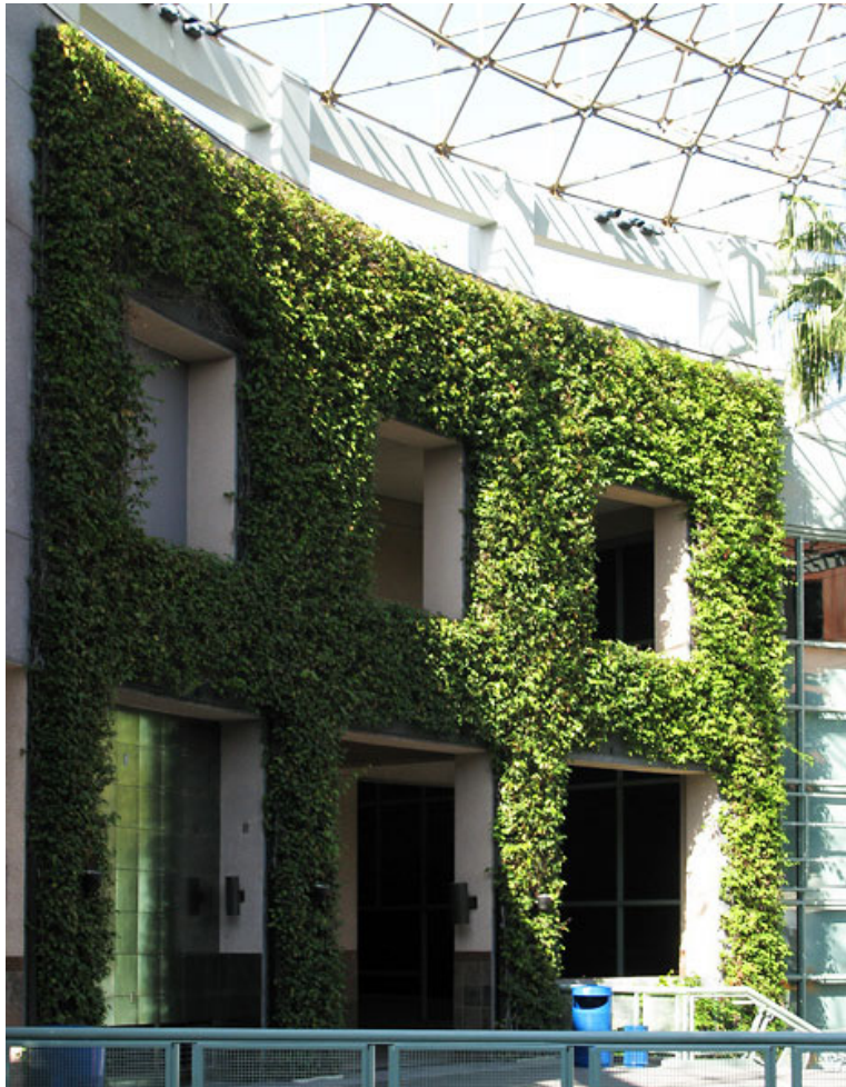
Proper soil volume, irrigation delivery and maintenance are successfully demonstrated in this 18-year-old green facade installation, Universal City, CA.
