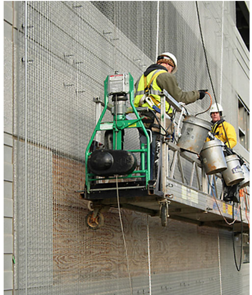
Matching contractors with appropriate scope of work and equipment will help alleviate installation issues, Riverdale, MD.
