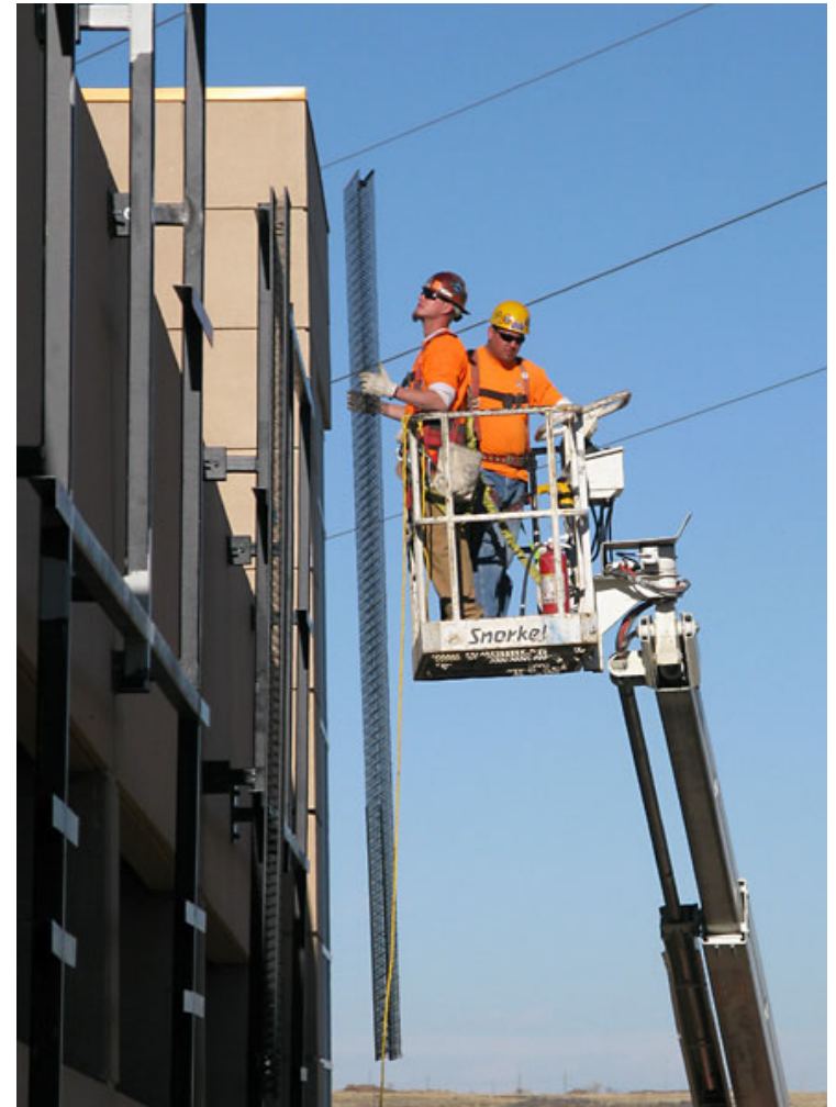
Rigid, lightweight, three-dimensional panels being installed on a multi-level building, Golden, CO.
