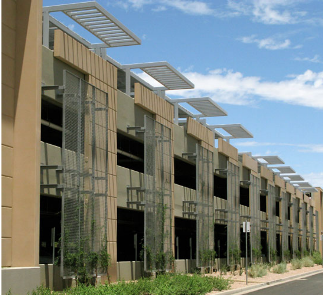
Inspection of system components and plant material is crucial for proper specification enforcement, Tempe, AZ.
