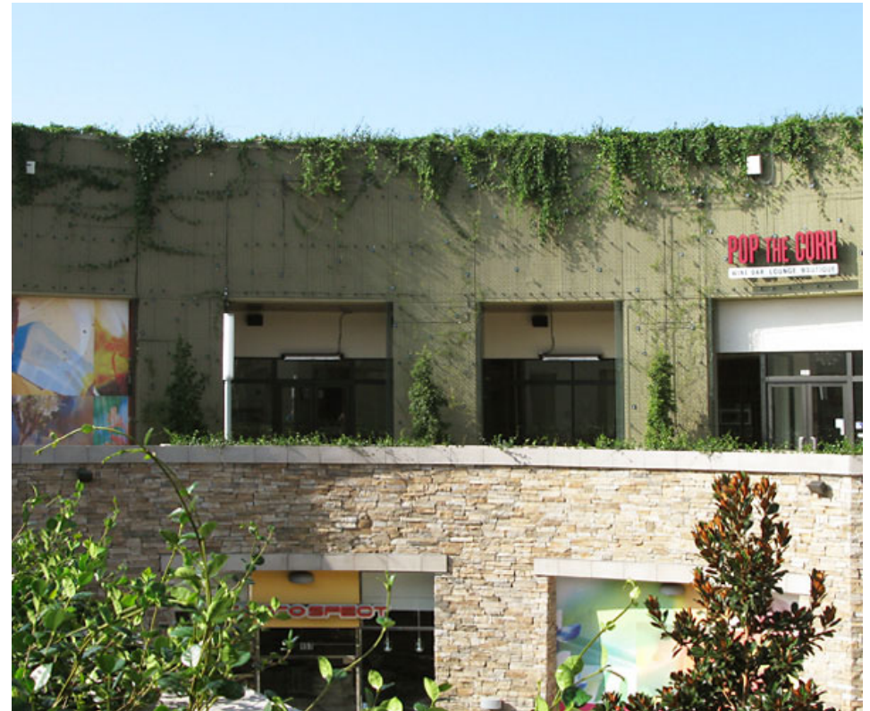
Green facade mounting connections are located where appropriate structure is available to cover large surfaces and for surrounding openings, Anaheim, CA.
