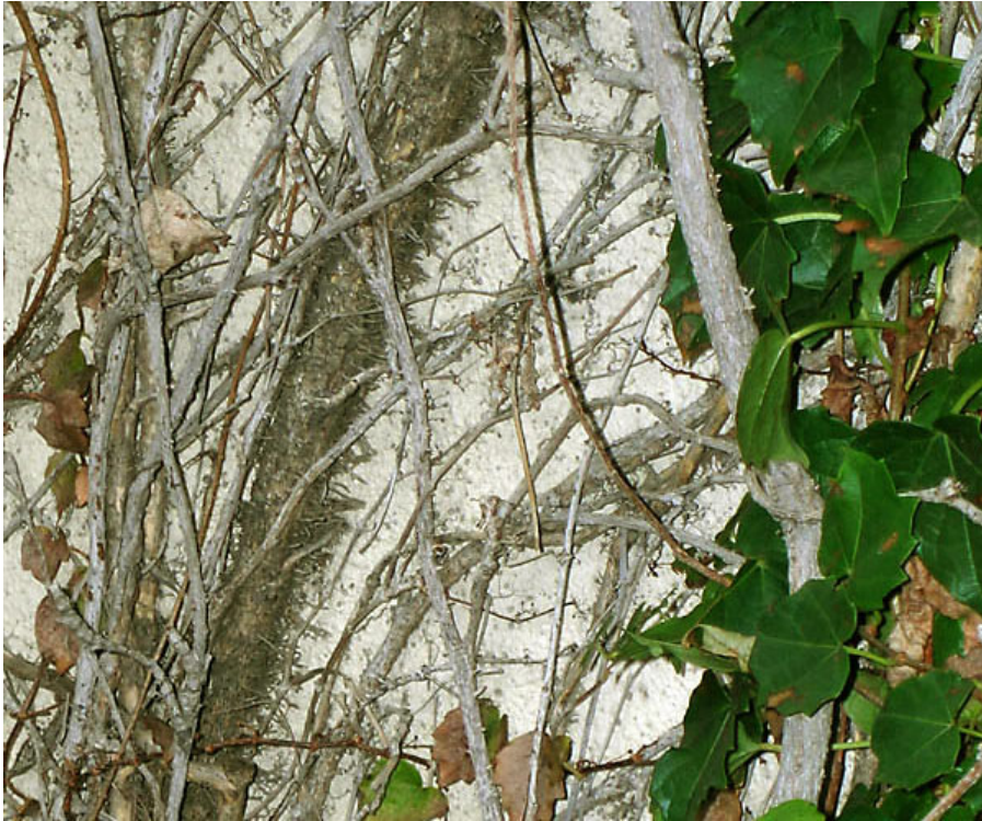
Aerial root species attached to the building surface.
