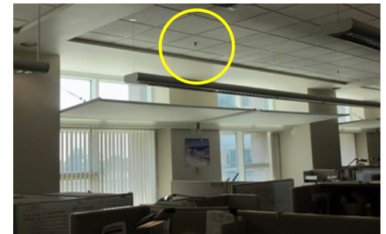
Light shelf directly below sprinkler head
