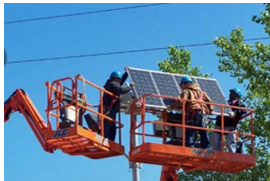
Distributed Solar Lighting
