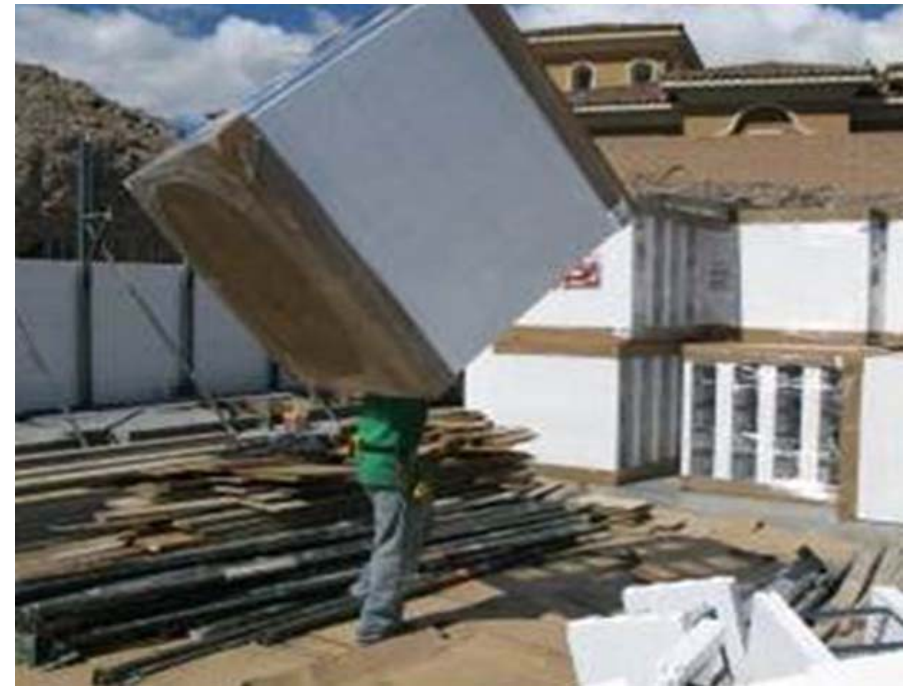
ICFs are much lighter than traditional reusable form systems. This photo shows one man handling a bundle of ICFs.
