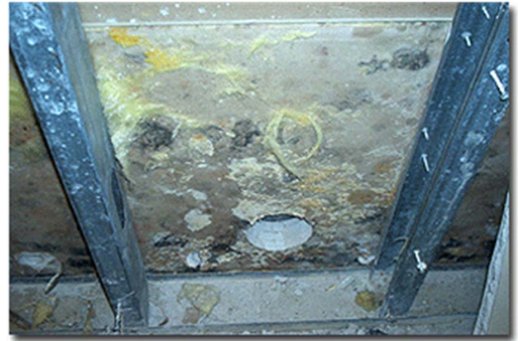
Mold in wall cavity
